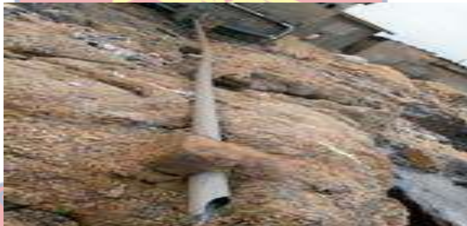
Figure 10: A tube to discharge public toilet waste into the sea at Moree Source: Anokye (2020)
