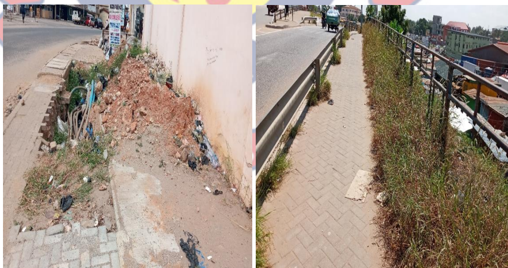
Figure 9: Showing an unclean and cracked walkway in Adabraka and Achimota overhead
