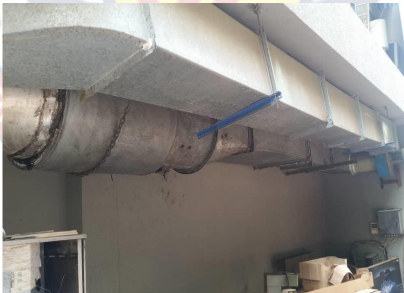
Plate 9: Ventilation Hood in a Hotel Restaurant Kitchen
