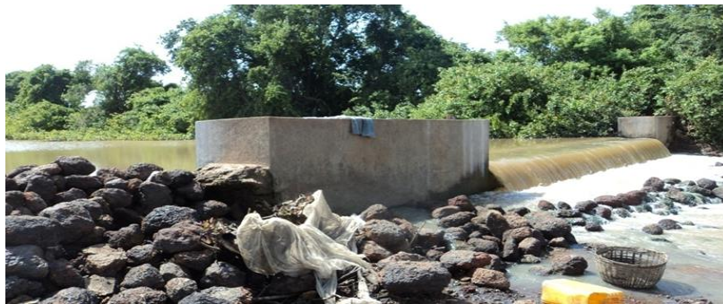
Plate 26: A gabion constructed at Nabogo wetland to correct an incised channel along the course of the flowing water
