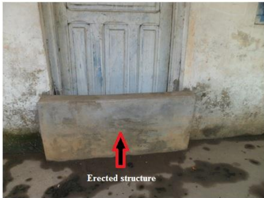
Plate 6: Erected structure in front of a door to prevent flood waters from entering the room
