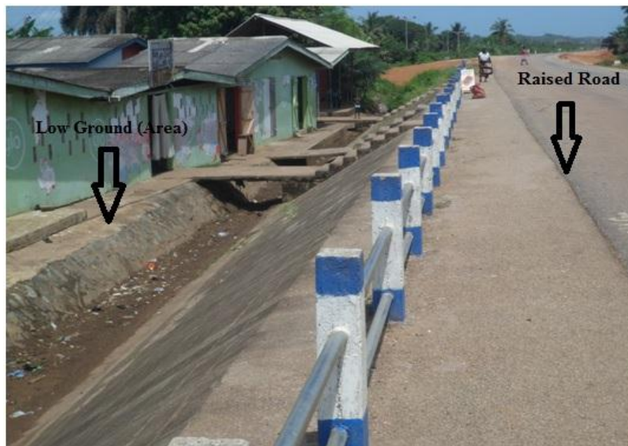
Plate 2: Axim- Elubo road through Asanta which causes flood
