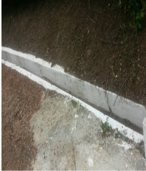
Figure 6: Image shows open gutter at Akropong School for the Blind.
