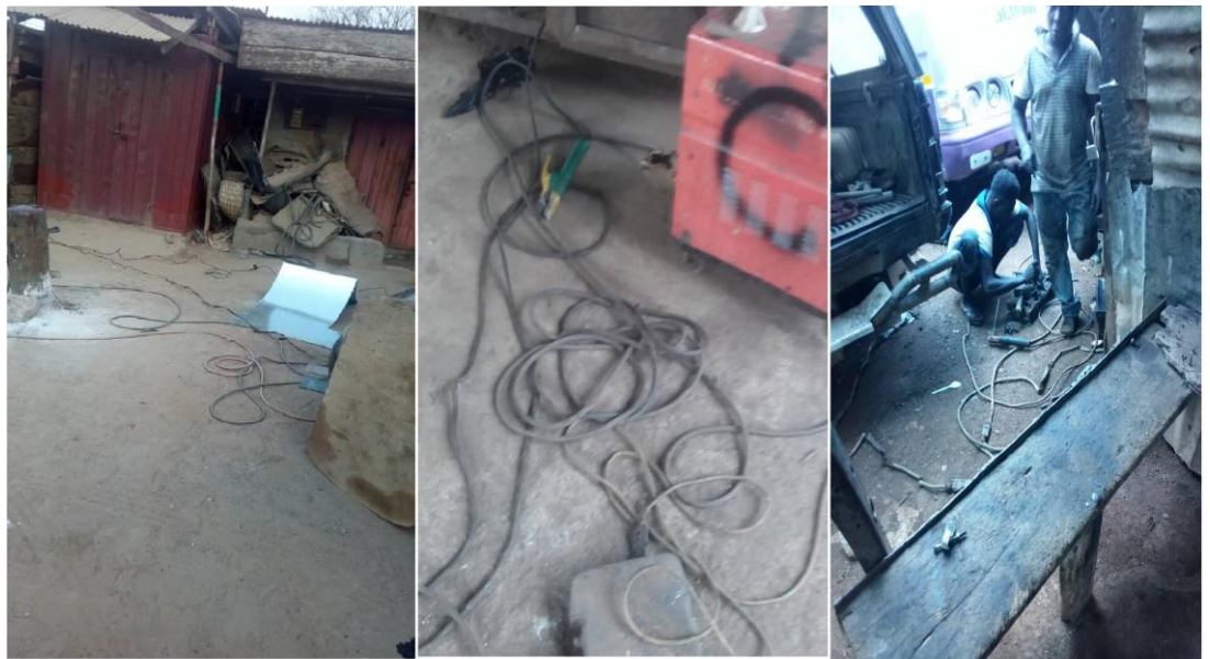
Figure 9: Electrical wires strung across walkways in a workshop
