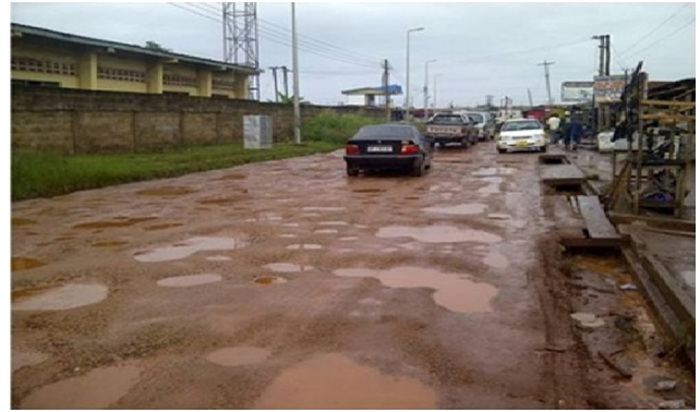
Fig. 2. An image showing one of the poor roads in Ghana Figs 1 and 2 [20].
