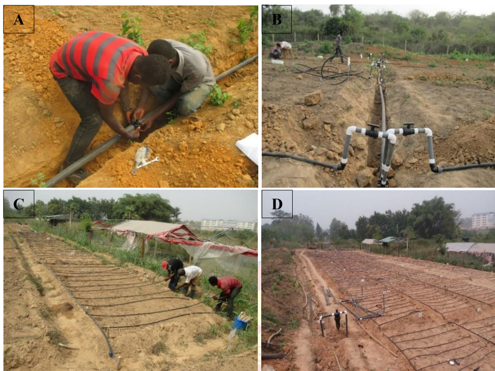
Figure 3.5: Installation of drip irrigation kits on the experimental plots. (A): Fixing of sub-main line, (B): flushing valve connected to the sub-main line and flushing manifold, (C): connecting dripper lines to the flushing manifold and (D): installed drip irrigation kits connected to a filtration unit.
