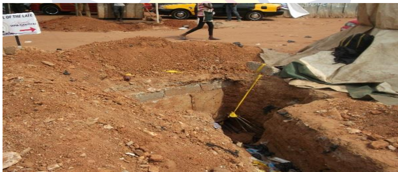
Figure 19: Pedestrian walkway cut-in by utility companies impeding free flow of walking
