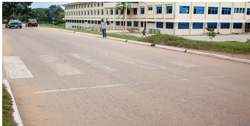
Plate 1: Faded Pedestrian Crossing Site
