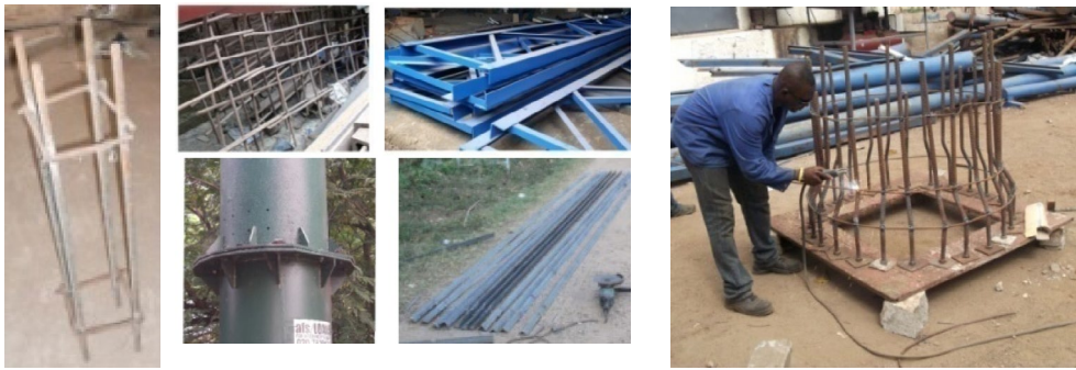
Hold down bolt Joint of two poles Angle Irons Construction of holding down bolt
