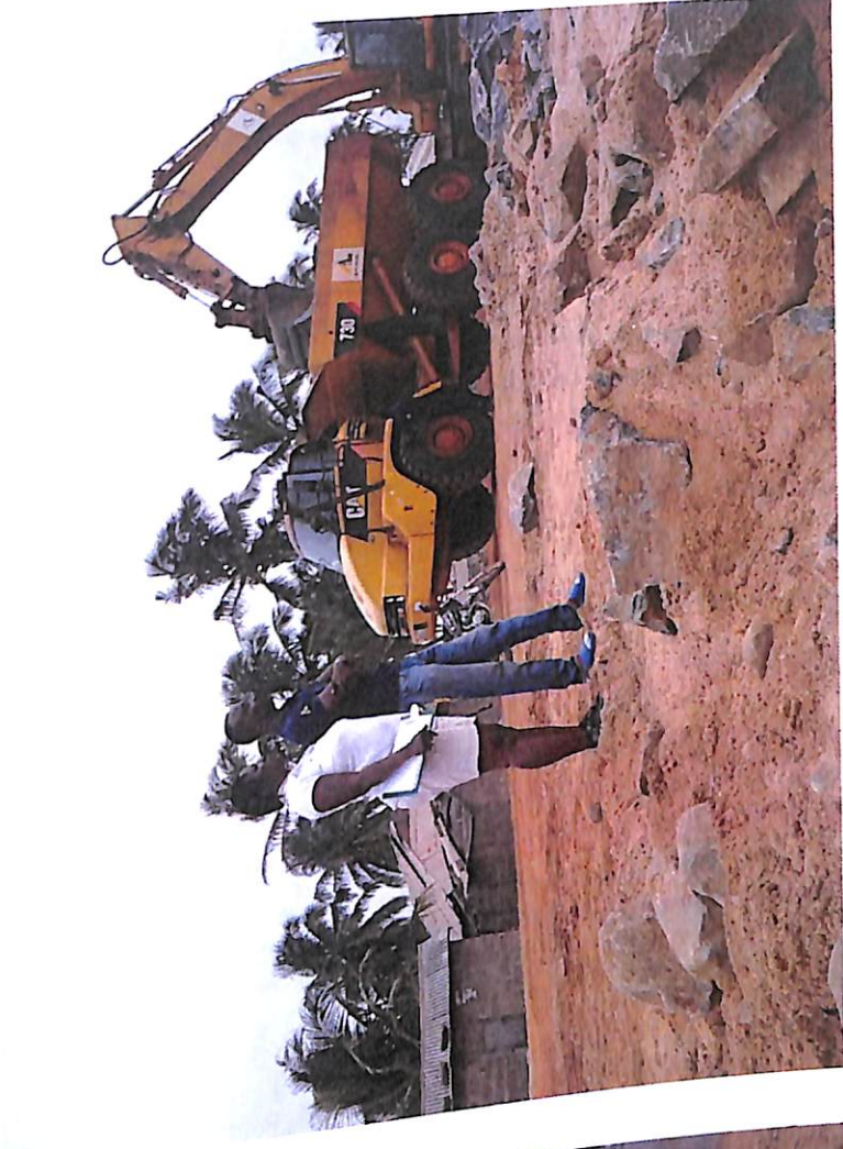
Figure showing the construction of new CES at Blekuso due to erosion being caused at downdrift side of the Kedzi-Keta structures by AMANDI
