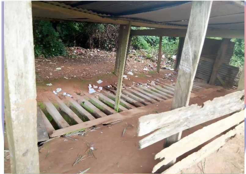
Figure 16: State of latrine for pupils at Nyamebikyere D/A Basic Source: Field survey, Otami (2019)
