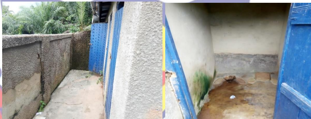
Figure 14: Latrine and Urinal for pupils in Odoben Amafua D/A Primary
