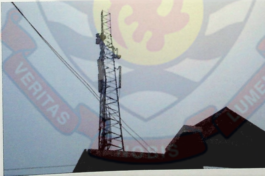
Plate 8: Typical Roof Top Tower at site H
