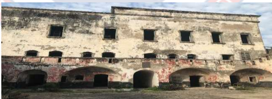
Figure 9: The Paint of a HA Peel off Source: Fieldwork, Koufie (2021)
