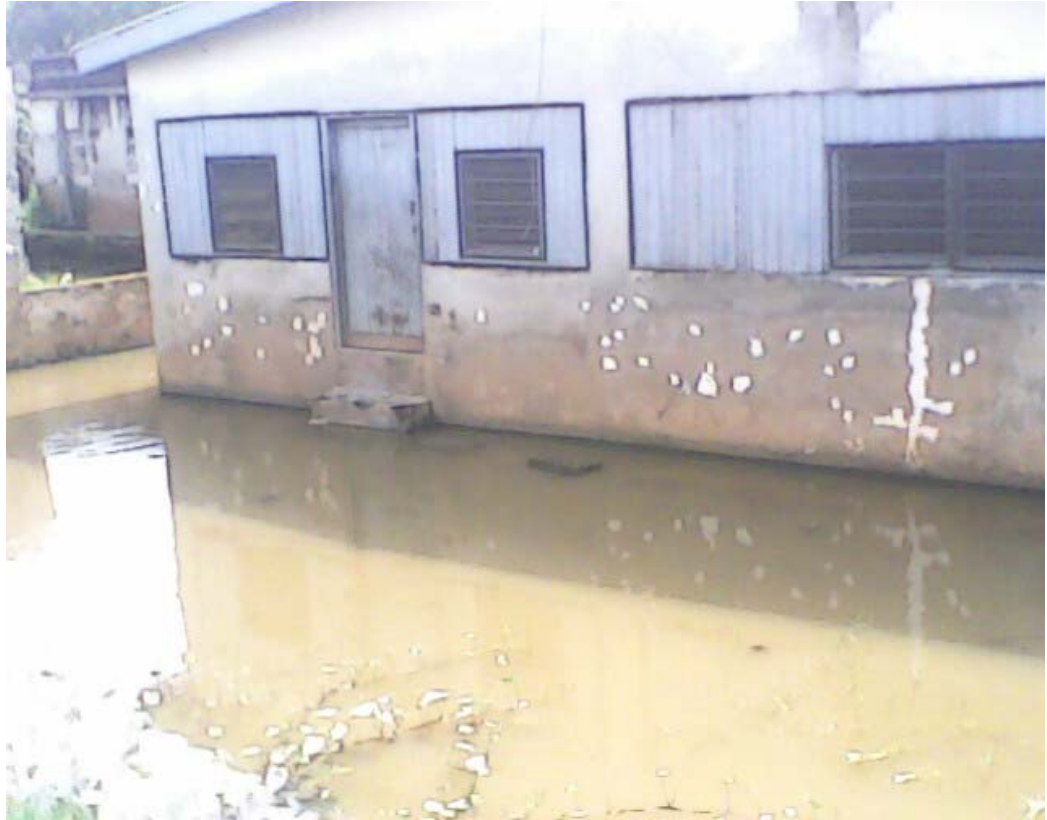
Plate 5: Evidence of flooding at Aboabo
