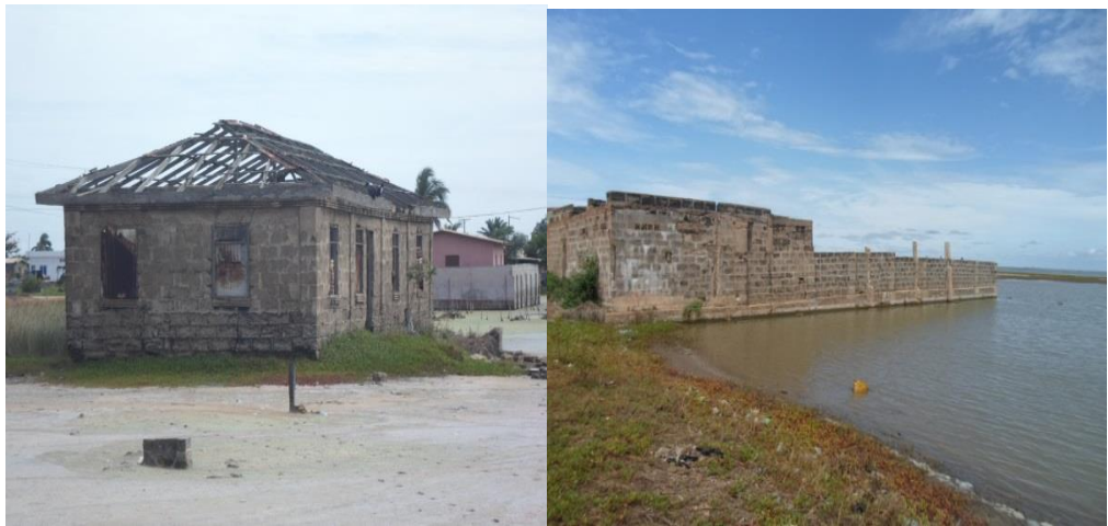
c. Abandoned uncompleted buildings near the lagoon
