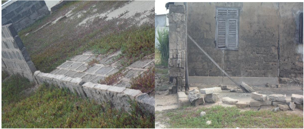
b. Collapsed walls and exposed foundations near the lagoon
