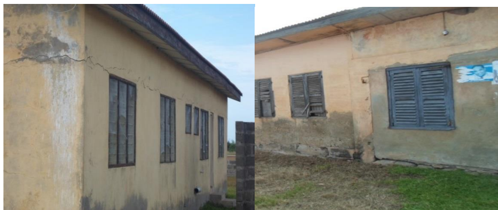
a. Cracked building near the lagoon
