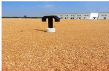
Air vent on top of the storage tank
