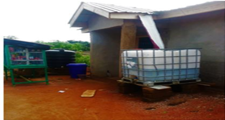
Water tanks for storing water connected to rain gutter for harvesting rainwater
