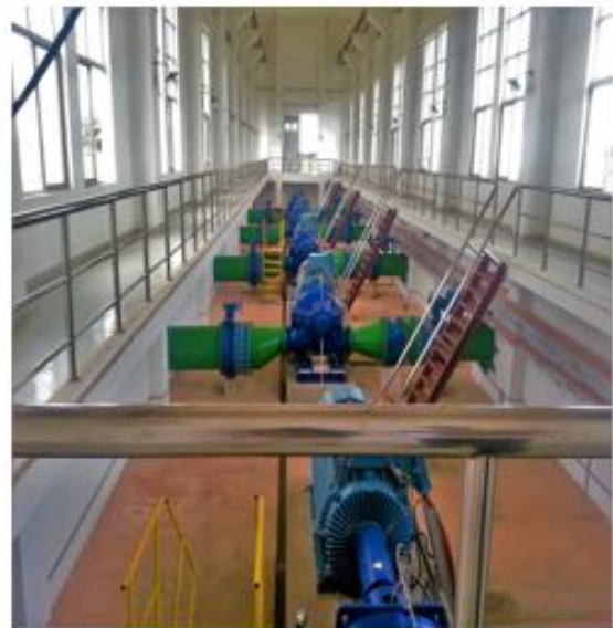
Pump station where water is pumped from the tanker to another station.
