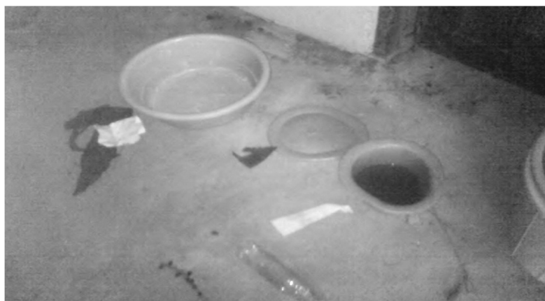
Plate 2. The floor of the toilet room in Basic School A
