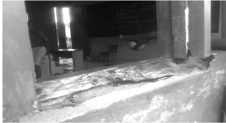
Plate 5. A broken classroom window in Basic School A
