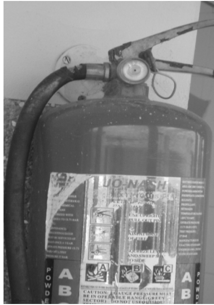
Plate 21. Fire extinguisher in Basic School B
