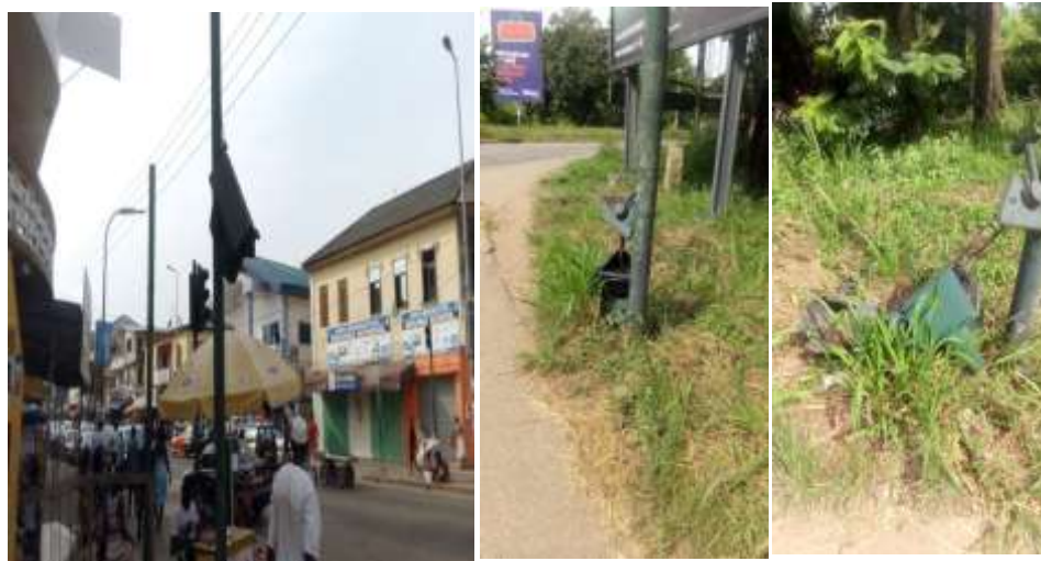
Plate 7: Broken down Traffic Lights in the Metropolis
