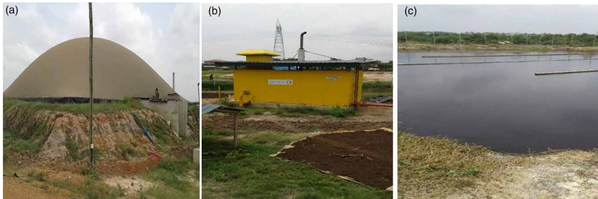
Figure 7 | (a) The Safisana fixed dome biogas plant, Ashaiman, Accra, September 2017, (b) the CHP at the Safisana Ashaiman site, September 2017; (c) Waste stabilisation pond with baffles at the Ashaiman site for treatment of liquid waste from the drying beds, September 2017.
