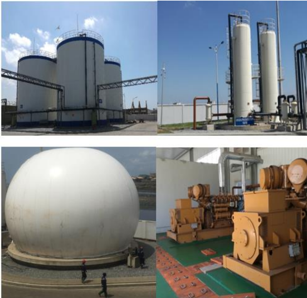
Figure 6: Overview of the Biogas to Electricity intervention; this is being used at Lavender Hill FSTP
