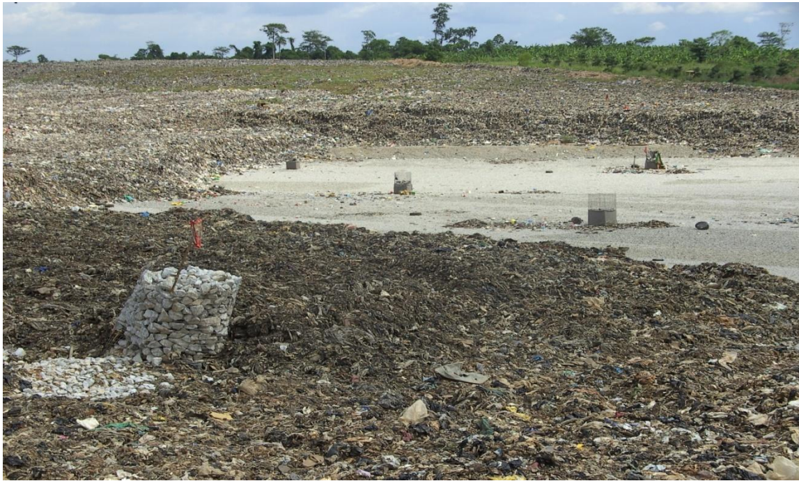
Figure 2. Seams for future flaring of gas covered with solid waste
