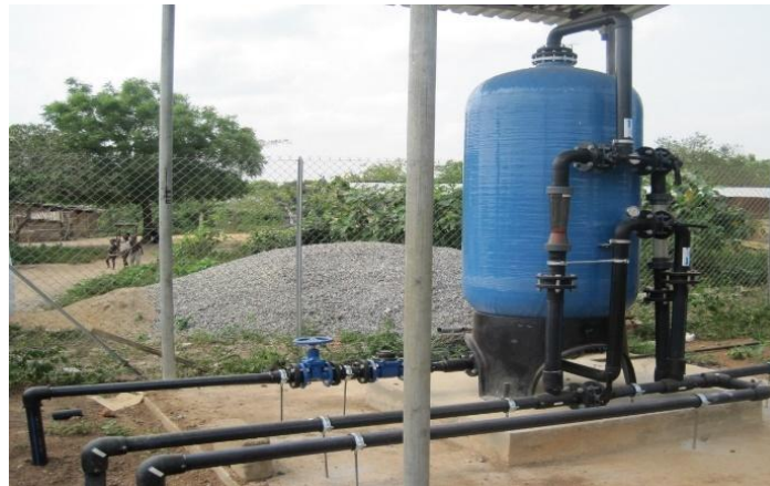
Plate 2. An Aquatec filtration unit installed in the AFSTWSS (Source: ANMA [20])
