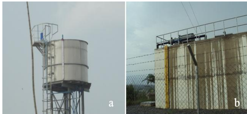
Plate 3. Service reservoirs of the AFSTWSS (a) Elevated aluminium reservoir; (b) Ground-level concrete reservoir (Source: ANMA [20])
