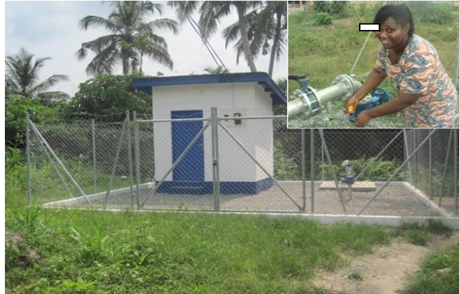
Plate 1. Water source – borehole and pumping station – at Assin Fosu (Credit: Authors)
