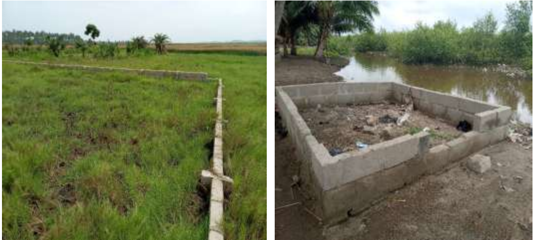
Plate 6: Structure being put up within at the north eastern and southern section of the wetland area.
