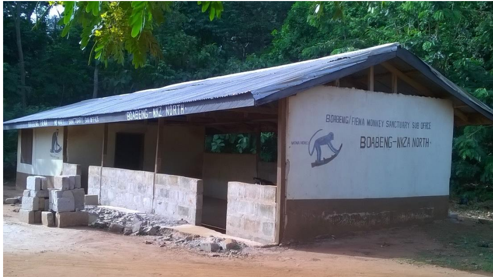
Figure 23: BFMS Guest Reception Centre 2, Partially Damaged During a Youth Demonstration over Poor Accountability.
