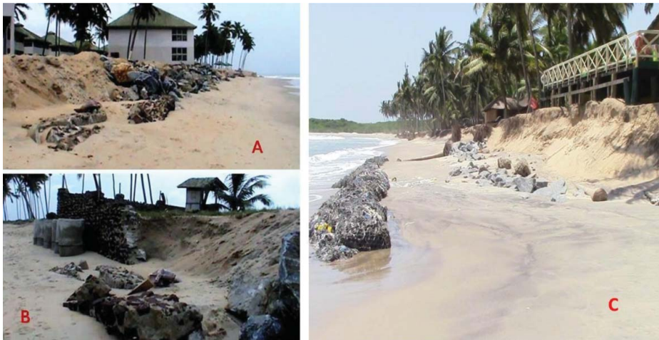
Figure 6. Examples of degraded small scale beach front sea defence projects along the Elmina–Cape Coast–Moree area of Ghana, (A) and (B) are in Elmina, (C) Erosion is near Cape Coast.
